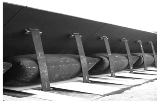
Obermeyer gate structure showing inflatable bladders.
